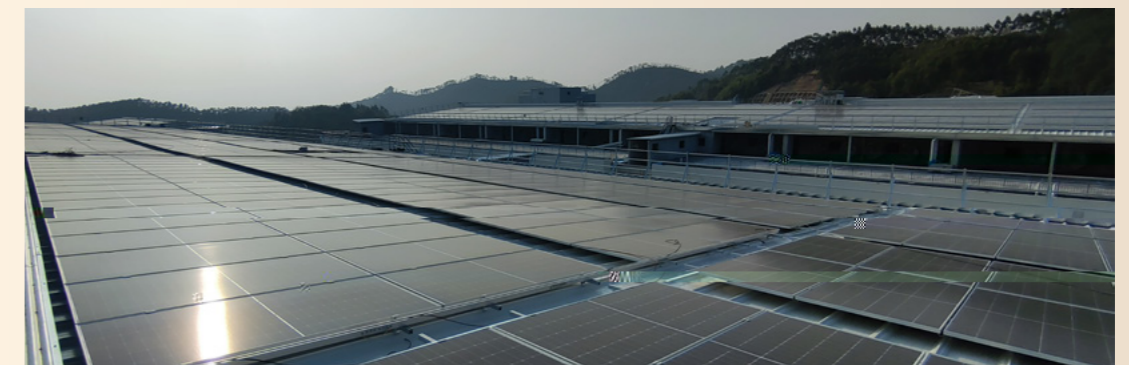
Yuexiu Capital PV Project
